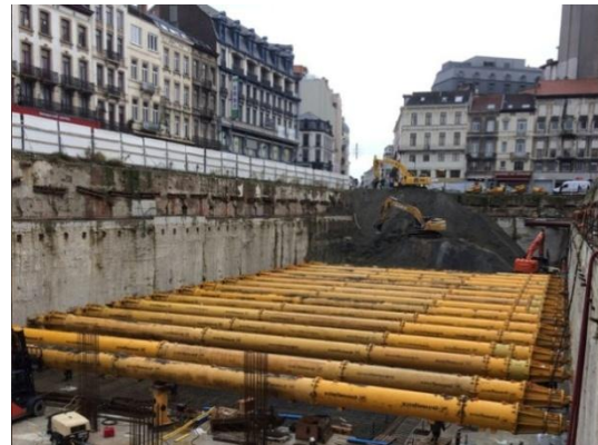
Google Fair Use Hydraulic struts between the side walls of an old parking lot during the BruCity construction site in Brussels.
