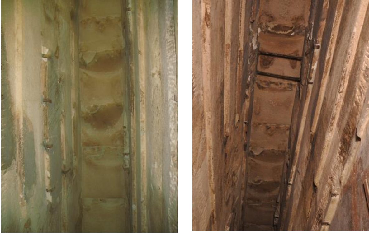
On the left, photo from 2005, on the right, photo from 2017. The successive semicircular aureoles are visible on several roof slabs, the first two being more marked than the following ones. On the photo on the right, the stains in the upper part are random.
