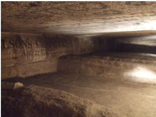
Empty space called "Nelson's room" between the beams/struts of the 2nd and 3rd "ceilings" which sink about 1m into the North and South side walls.
